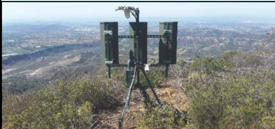
AE6XE Orange County, California 3 node installation Photo Credit: AREDN
